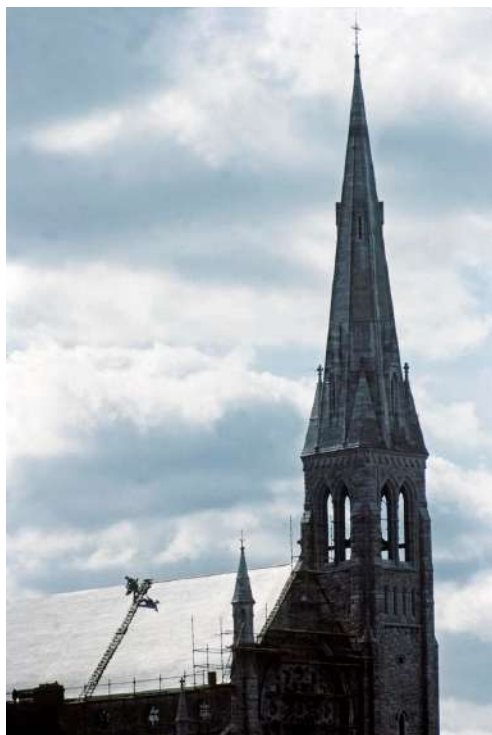
UC:P351/3/P1/200: County Limerick, Kilmallock, a man at work on the roof of the church, 1984.
